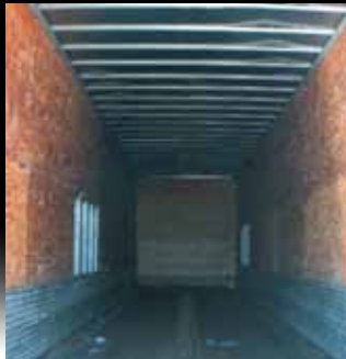
Typical interior damage from daily loading and unloading
